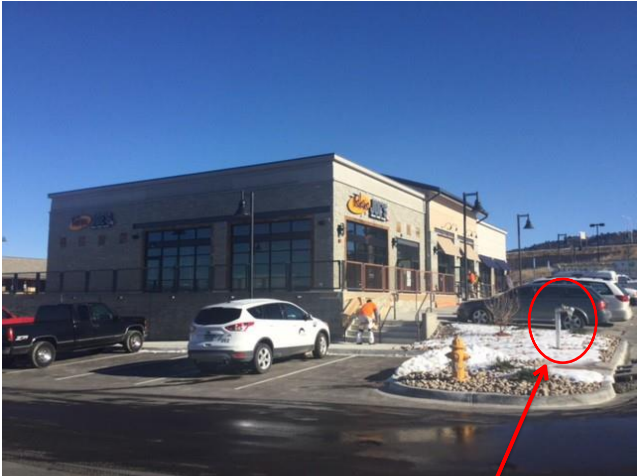
Completed FDC located near a hydrant, away from the building accessible to the fire department
